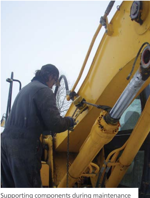
Supporting components during maintenance
